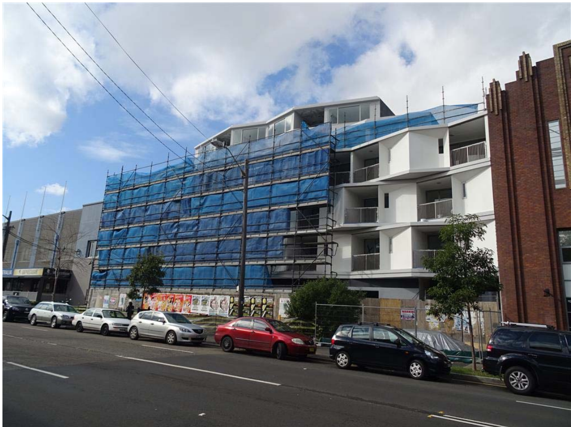
Figure 10: Shop top housing under construction on the opposite side of Botany Road.
